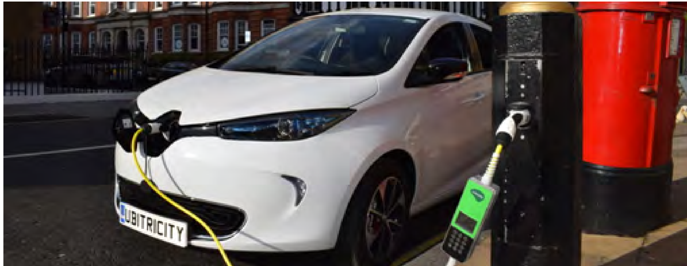
Figure 60. Electric charging point integrated with street furniture.
