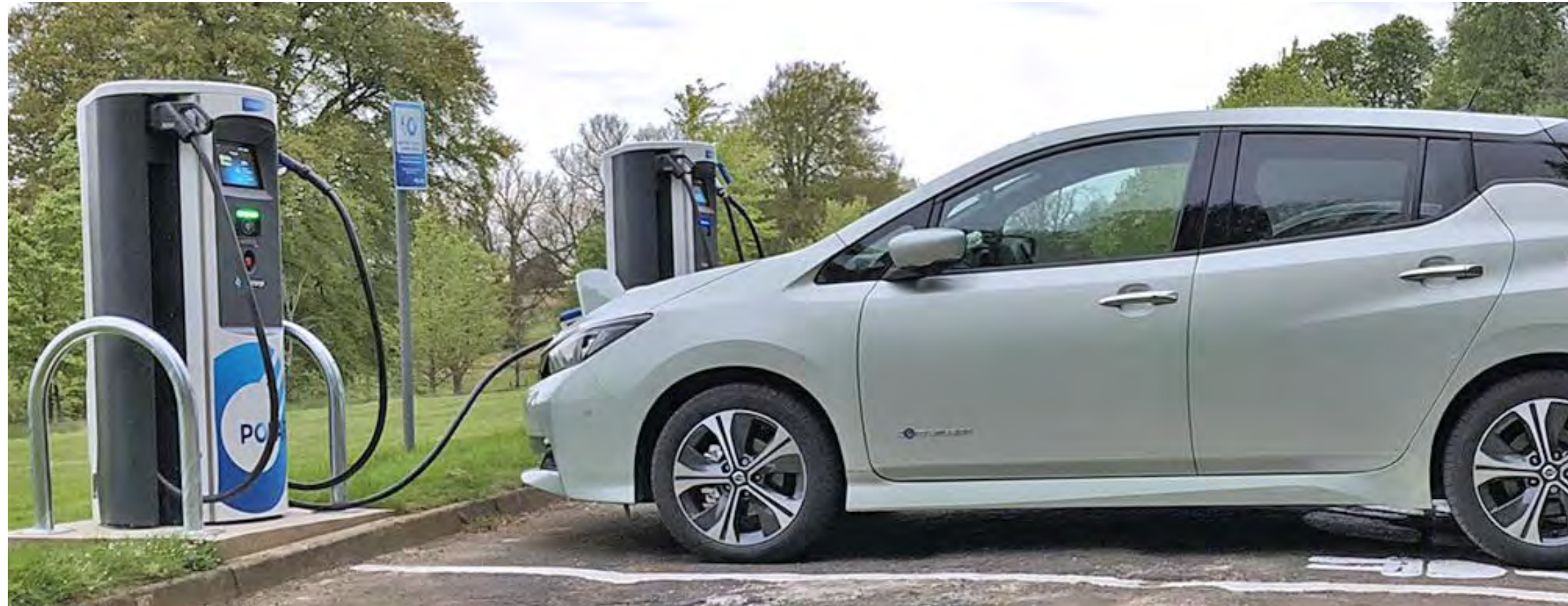
Figure 59. Electric charging point for vehicles.
