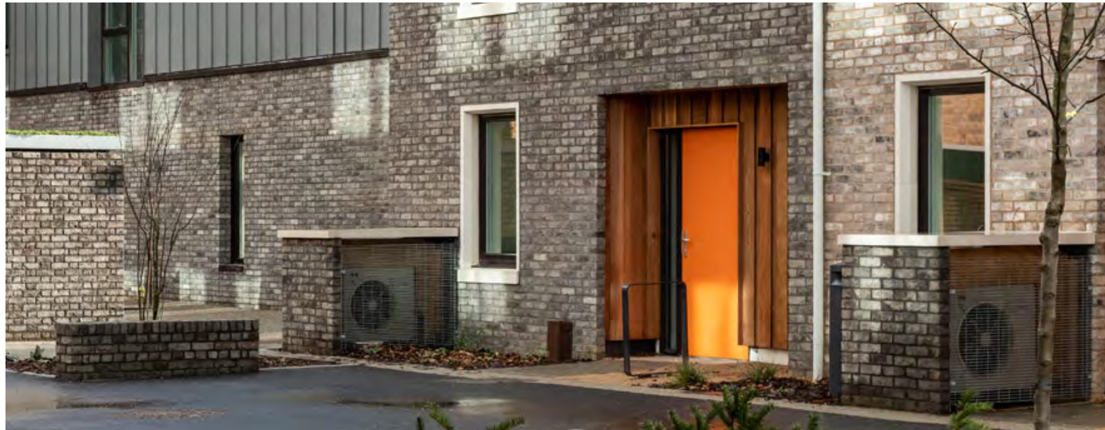
Figure 57. Air Source Heat Pumps
